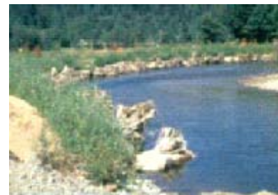
Figure 8.47: Completed system after one year. Note dramatic willow growth from vegetated geogrid.
