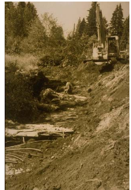
Figure 9.7: Backhoe in operation at a restoration site. Backhoes are mobile in rough terrain and can move rocks and logs with remarkable precision.
