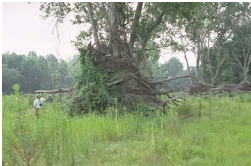
Figure 9.16: Flood debris. The entire corridor should be inspected annually to detect areas of debris accumulation from flood flows.
