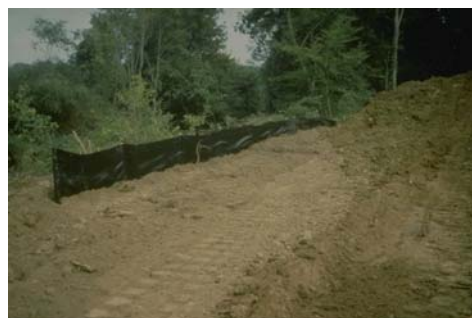
Figure 9.2: Silt fence at a construction site. Properly chosen and installed silt fences can provide a significant degree of off-site sediment control.
