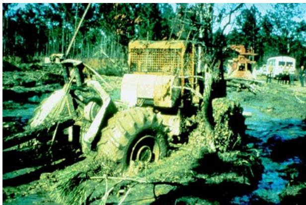
Figure 9.9: Lessons to be learned. Heavy equipment can quickly reduce a vegetated area to churned earth.
