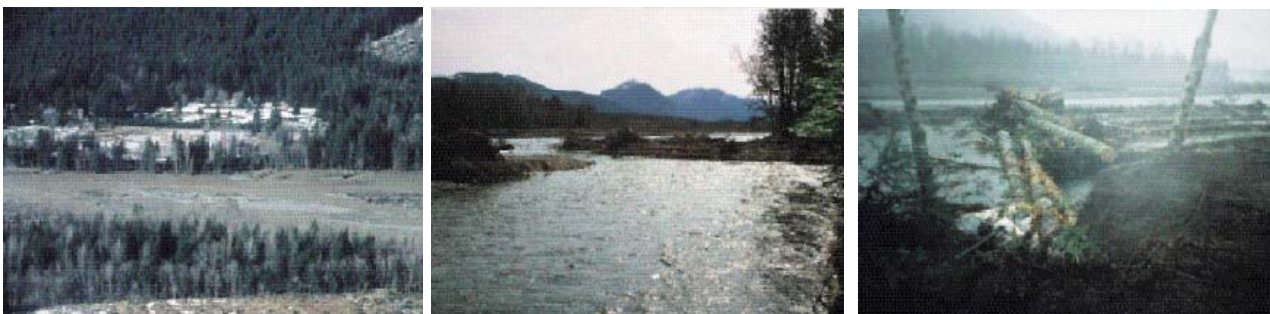
Fig. 9.23: Engineered log jams. Engineered log jams (ELJs) can restore riverine habitat and in some situations provide effective bank protection.
