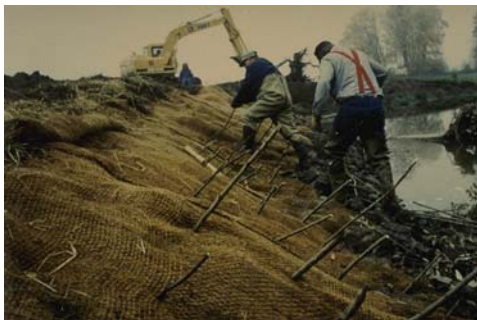
Figure 6.7: Installation of erosion control fabric. Installing measures can be considered a "mid-point" in restoration and not the completion. Preceding installation is the necessary planning, with monitoring and adaptive management subsequent to the installation.
