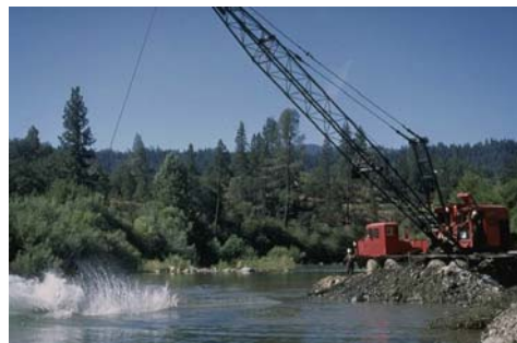
Figure 6.15: Instream construction activity. Site work in and around aquatic features is one of the most heavily regulated types of activity in the United States and should not be attempted without a sound knowledge of the relevant laws and regulations.
