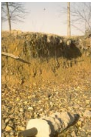
Figure 5.10: Streambank erosion. In designing alternatives for bank erosion it is important to assess the feasibility of addressing the cause of the problem (e.g., modify land uses) or treating the symptom (e.g., install bank-erosion control structures).
