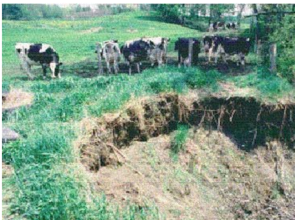
Figure 6.24: Streambank failure. Midcourse monitoring will guard against unexpected damages.
