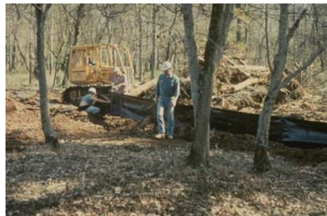
Figure 6.14: Workers installing a silt fence. Familiarity with on-site conditions is critical to successful implementation of restoration measures.
