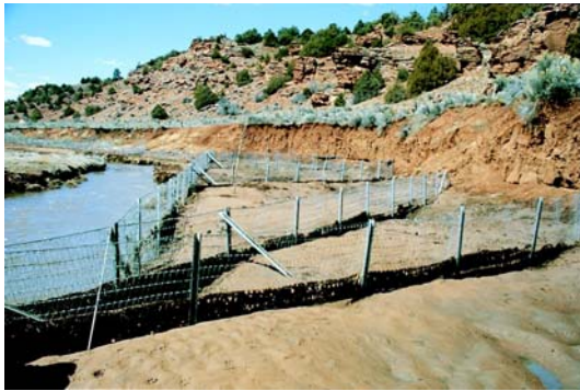
Figure 4.17: Recently installed treatment. (April 1987.) Porous fence revetment designed to reduce bank failure.
