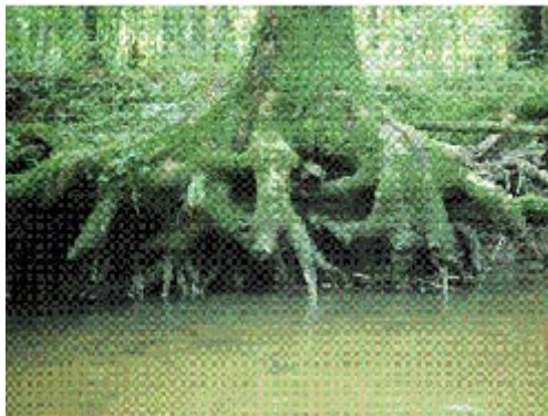
Figure 7.28: Bank erosion by undercutting. Removal of toe slope support leads to instability requiring geotechnical solutions.
